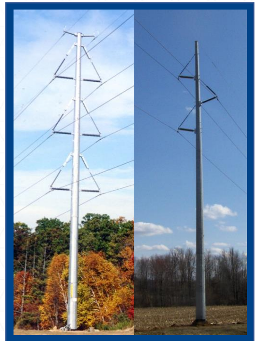
The new Long Rapids transmission line towers will be similar to the ones shown here. On the left is a double-circuit tower, and on the right is a single-circuit tower.
