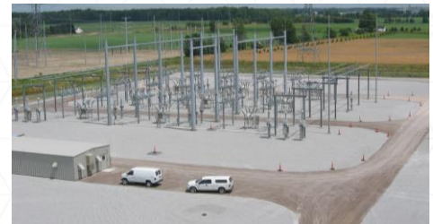
The new Shale Substation will be similar to the one shown here.
