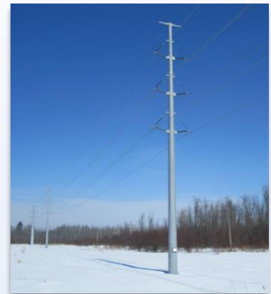
The new Garfield Avenue – Hemphill structures are similar to the one shown here.
